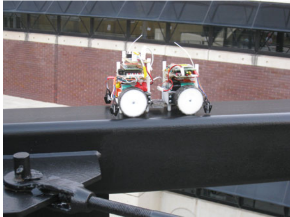
Fig. 11.3 A mobile sensor prototype (developed by researchers at the Georgia Institute of Technology, USA) is crawling on a steel pedestrian bridge. (Photo courtesy of Prof. Yang Wang, Georgia Institute of Technology, USA)
